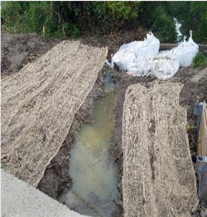
Fig 23: Jute netting installed on College brook slopes for restoration activities. Viewing west. (7-17-19).
