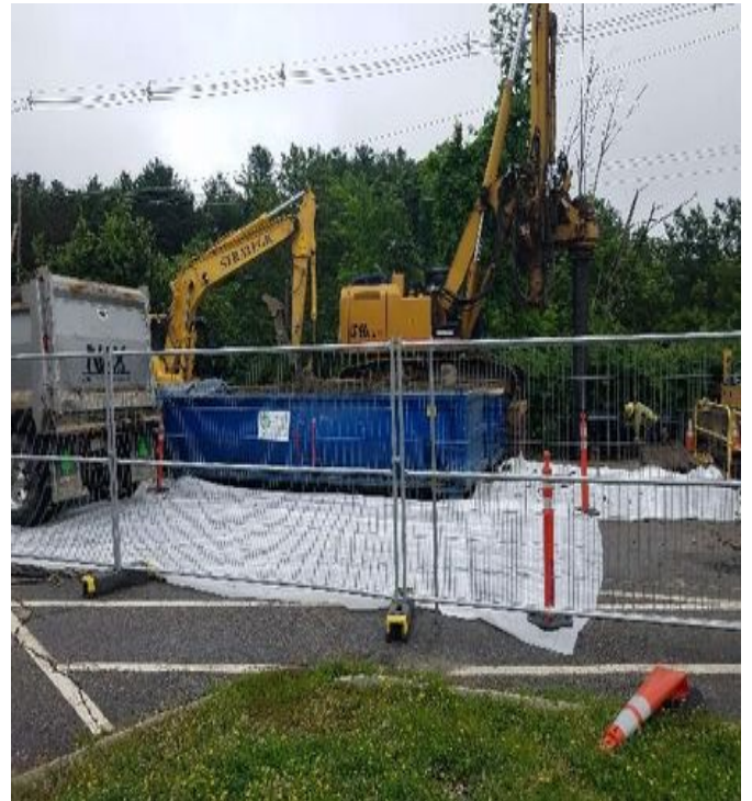
Fig 8: MJ drilling foundation for Str. 22, GZA has been managing the soil. Viewing east. (7-12-19).
