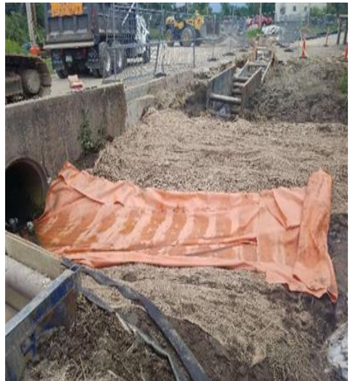
Fig 24: Filter fabric placed in the College Brook to help prevent sediment loss. Viewing south. (7-17-19).
