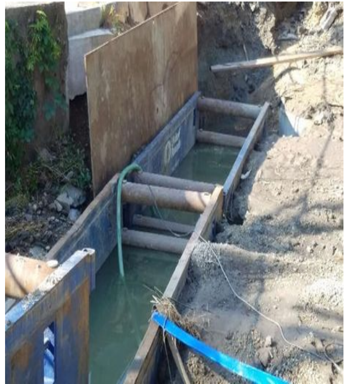
Fig 10: Rainwater in College Brook trench. Viewing south. (7-14-19).
