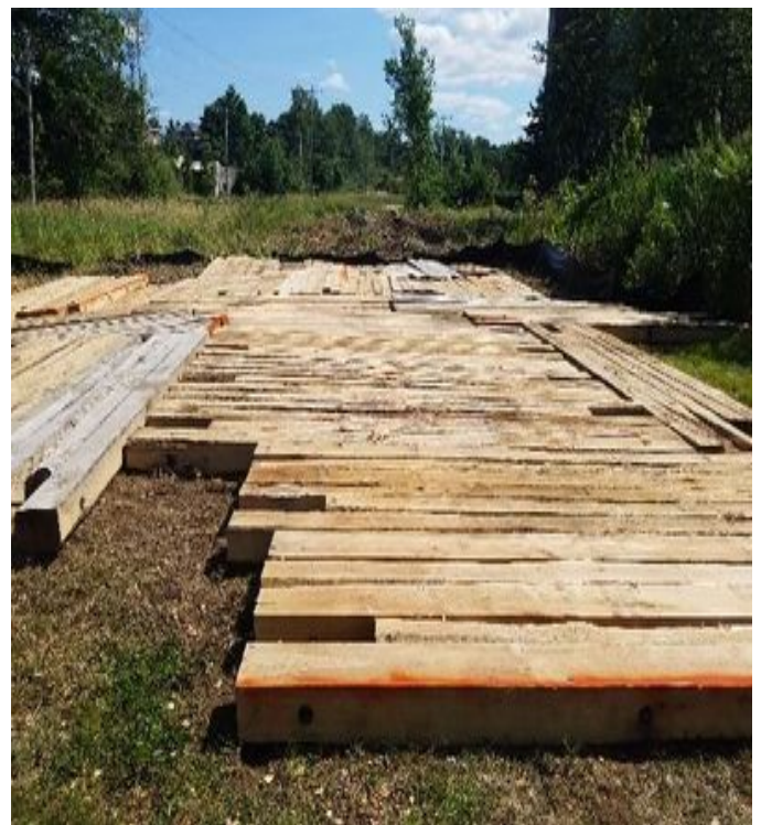
Fig 16: JCR began installing timber matting and erosion controls between Str. 23 and wetlands DW69 & DW67. Viewing south. (7-15-19).
