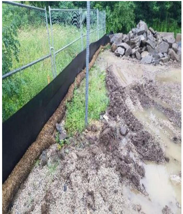
Fig 4: Erosion controls installed on the north side of the Waterworks Rd Laydown yard. Viewing east. (7-12-19).
