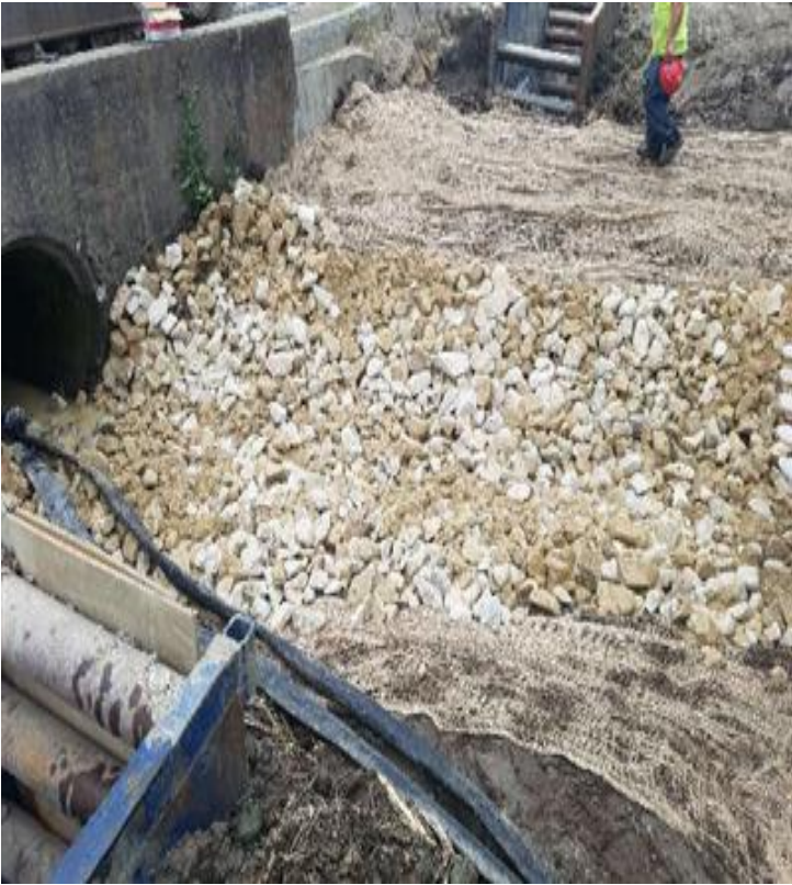
Fig 25: 6 in stone placed on top of filter fabric in College brook. Viewing south. (7-17-19).
