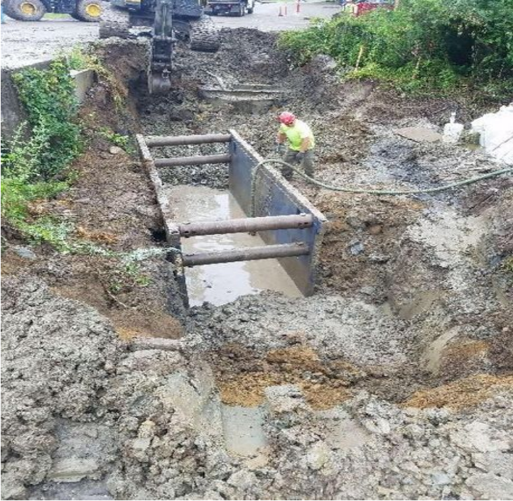
Fig 5: McCourt is pumping the trench water out and into the dewatering apparatus. Viewing south. (7-12-19)
