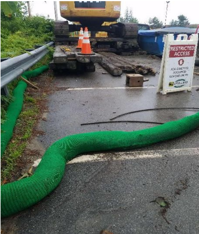
Fig 3: Filter sock installed around drilling activities for Str. 22 in "A" lot. Viewing south. (7-12-19).
